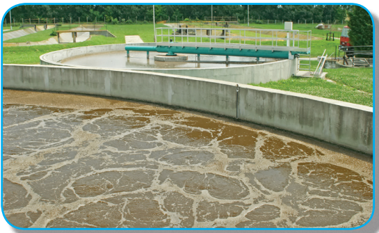
Waste Water Treatment
